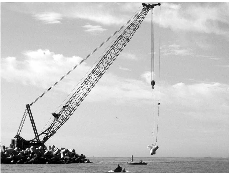
Figure 2. Activities conducted to expand the jetties in the Patos Lagoon Estuary. (A) Boat used to throw tons of rock to the seabed at the end of the jetties; (B) activity of throwing smaller rocks to the bottom of the sea by land when using trucks; (C) completion of work activities with the placement of tetrapods.
